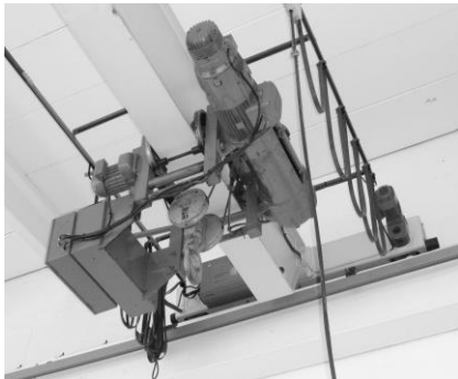
Figure 1 – Bridge crane at THGA
